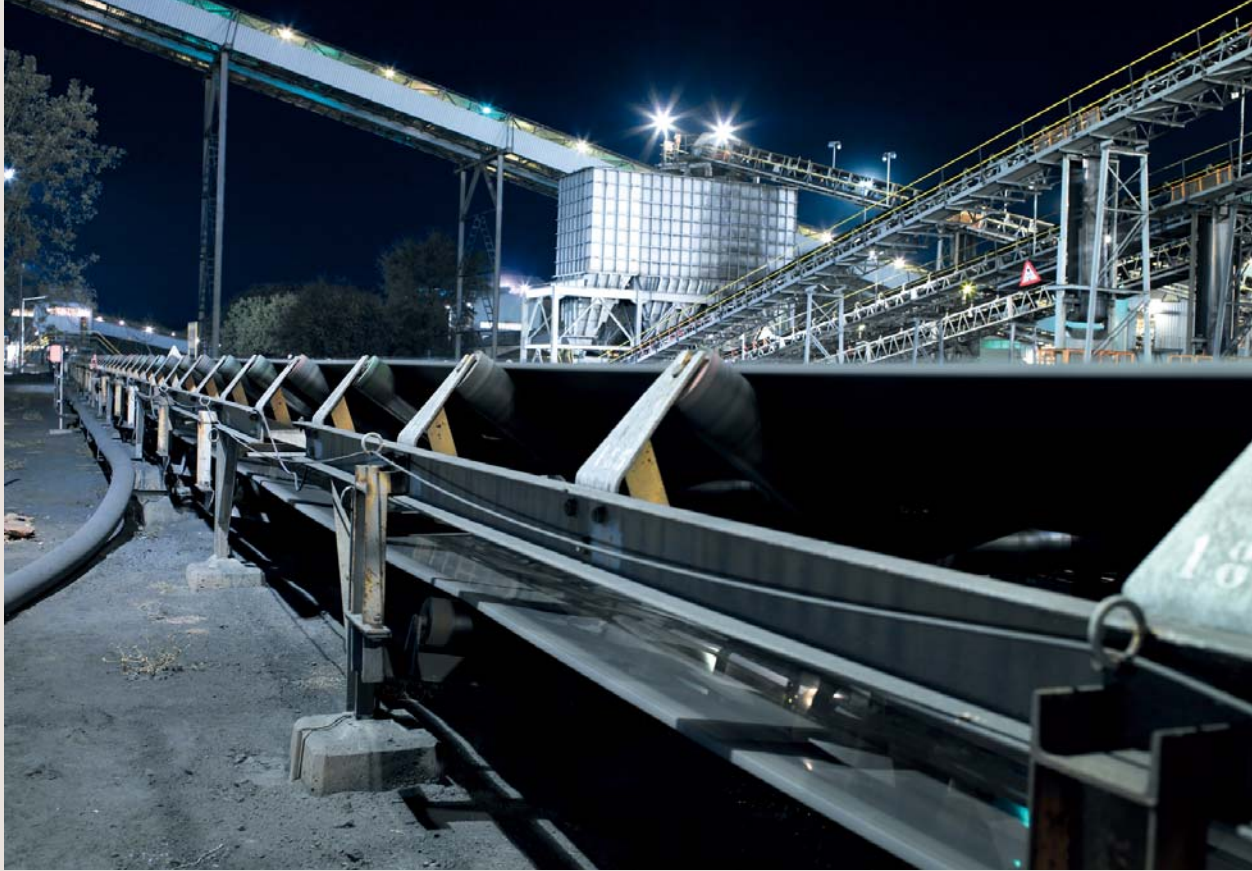
Beneficiation plant at Grootegeluk mine which produces power station, semi-soft coking and steam coal
