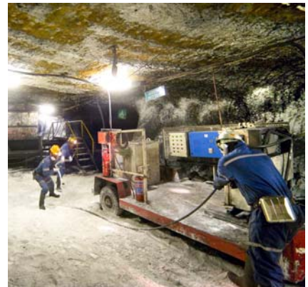
Underground power provision at Arnot mine, Mpumalanga
