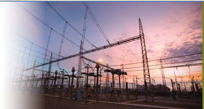
Apollo substation in Gauteng.
