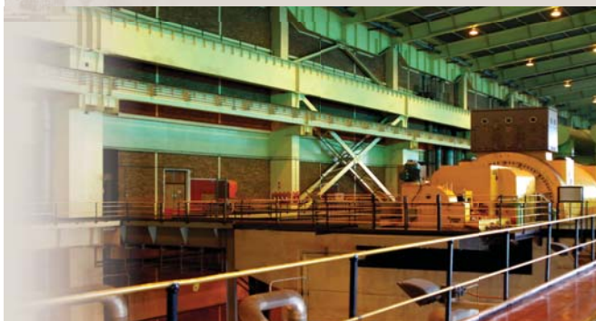
The turbine hall at Duvha power station near Witbank.
