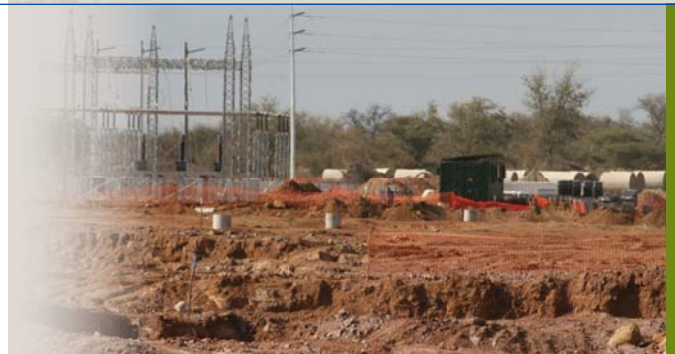
The new 132kV yard at the Medupi power station site.
